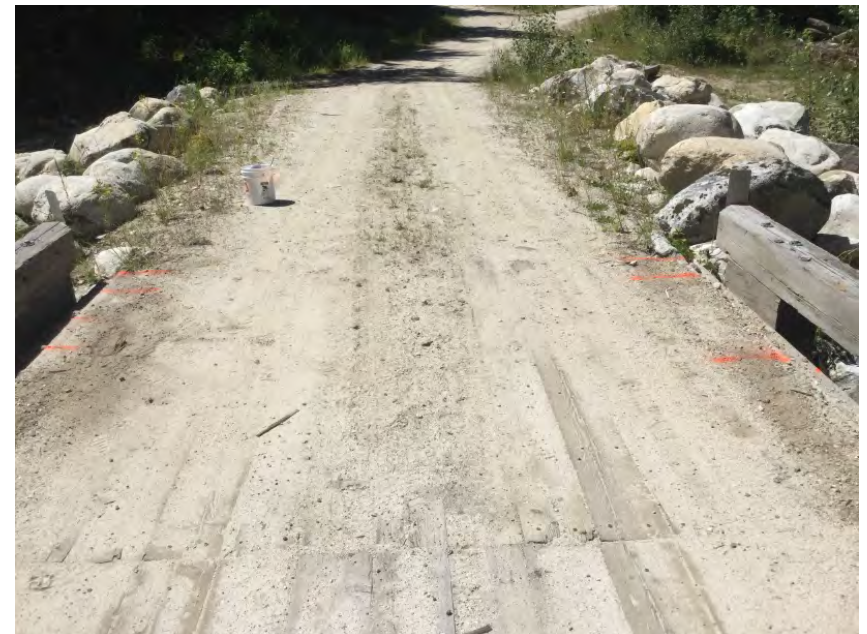
Rot Found in 5 Adjacent Ties at Right Abutment
