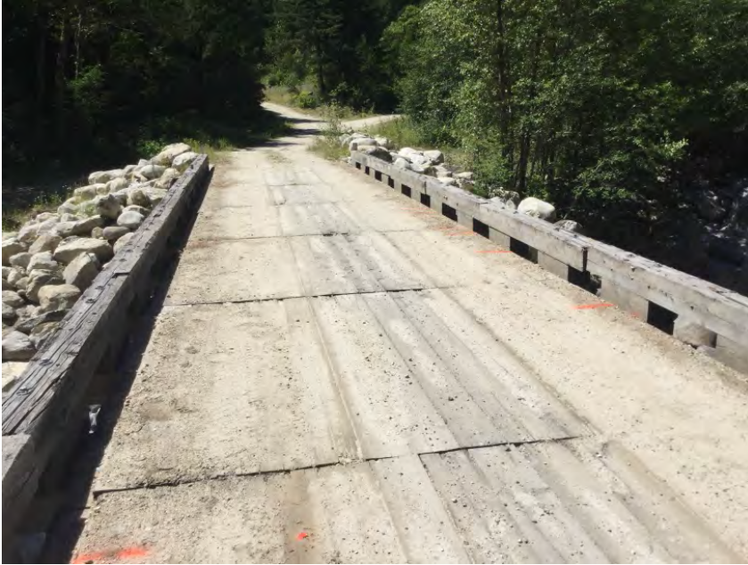
Rot in Ends of Ties Shown in Orange
